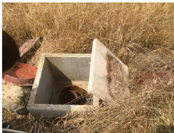
Well protection manhole
